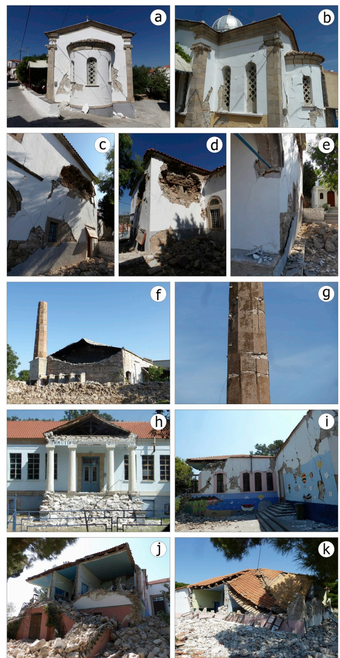
Fig. 10. Special structures including churches, industrial buildings and their masonry chimneys as well as schools suffered heavy damage from the 2017 Lesvos earthquake. Churches suffered damage including large cracks in various parts such as walls (a–e) and the dome, detachment of large pieces of plaster from load-bearing masonry walls (a, b, c, e), dislocation and fall of several roof tiles (e) and partial collapse of load-bearing masonry walls (c, d, e). Masonry industrial buildings in Vrissa suffered large cracks and partial collapse of their masonry walls (f) and large cracks of their masonry chimneys on the verge of collapse (g). School buildings suffered damage varying from fall of the gable over the main entrance (h) and cracks in their masonry walls (i, j) to partial collapse (k).
