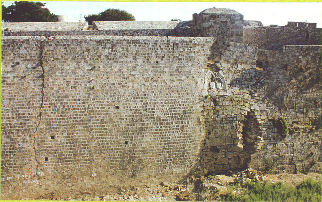
Fig. 6. Fracturing and bending of the structural elements of the Medieval Wall induced by differential subsidence movements in the vicinity of the F2 fault zone.
