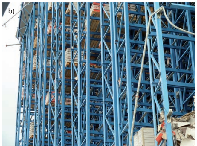
Fig. 18. a) A part of the ceramic warehouse in Sant' Agostino totally collapsed; b) This part of the same warehouse did not move. This can be very well justified by the relative position of the stored material to the steel members of the racks, which is in all positions the same. It must be taken under consideration that the positioning of the stored materials is computerized.
