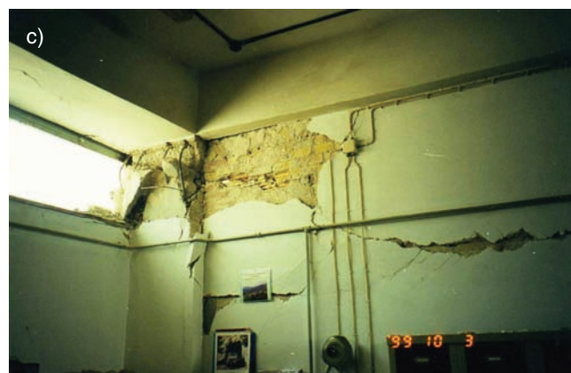
Fig. 29. "Short column", under a vertically propagated body wave action. The braking plane is perpendicular to the plane of the concrete wall and the respective beam. The adjacent window glass panel is unbroken. Not any significant residual vertical shortening is noticed. In c) the presence of a masonry wall perpendicular to the plane of the concrete wall did not prevent the break of the "short column".
