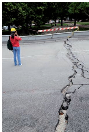
Fig. 14. Lateral spreading cutting through roads and residential area, in San Carlo.
