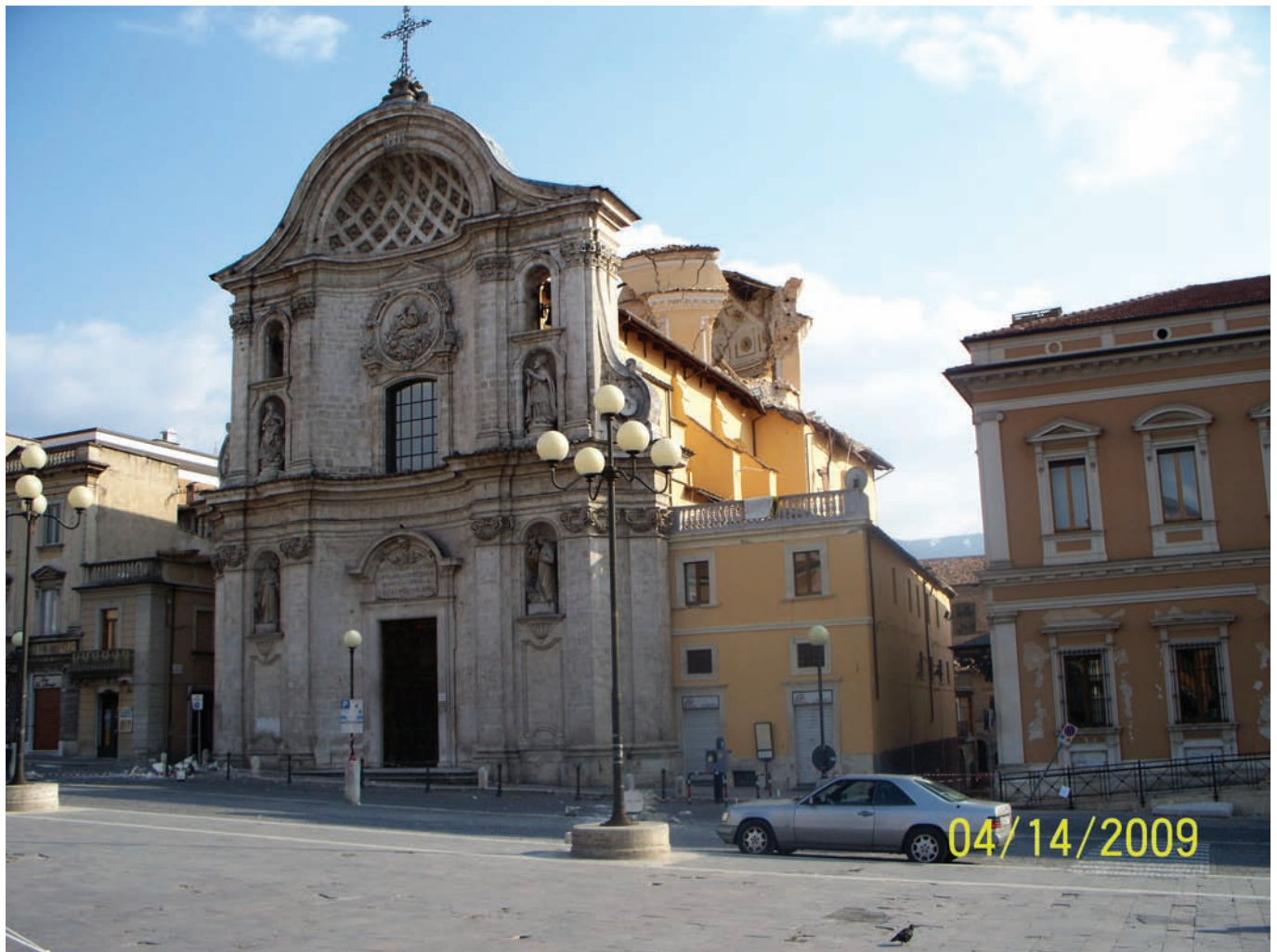
Fig. 27. Vertical collapse within the plan of the ground floor of the dome of Duomo church in L'Aquila, after the 2009 earthquake. There is not any other noticeable damage. Glass window panels are intact.
