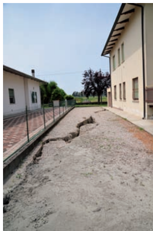
Fig. 13. Lateral spreading in San Carlo, with ejected liquefied grey fine sand material in residential area. Ground cracks with opening of about 20cm, vertical offset of 10-20cm and local extensional strains is evident.
