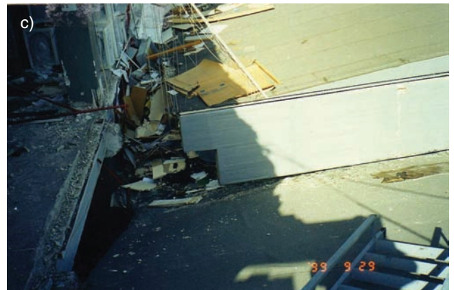
Fig. 31. a) Due to the vertical seismic component, the beam is jumping up and down on its supports if it is not sufficiently anchored; b) the corbel or the beam, or both are broken. In this case a vertical bolt is provided but it was too short and the beam jumped over; c) if there is a horizontal motion too, the results are worsened.
